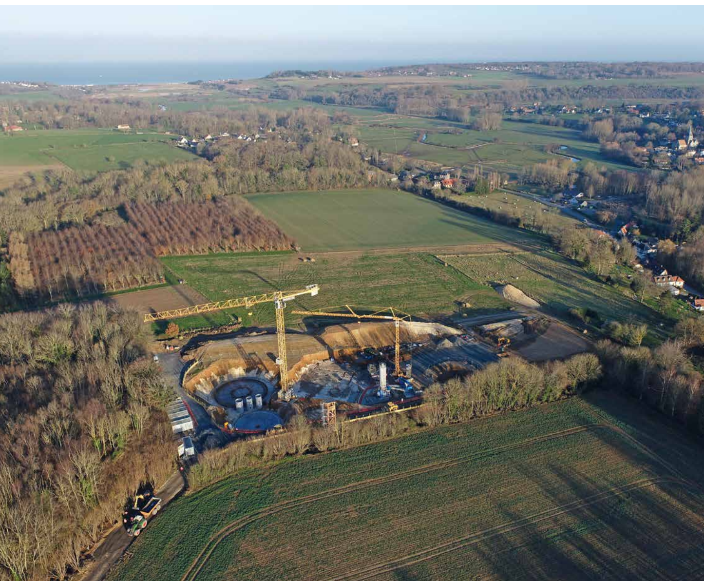
Figure 5. In Quiberville, a new, much larger sewage works is being built. Photo credit: Conservatoire du littoral.
