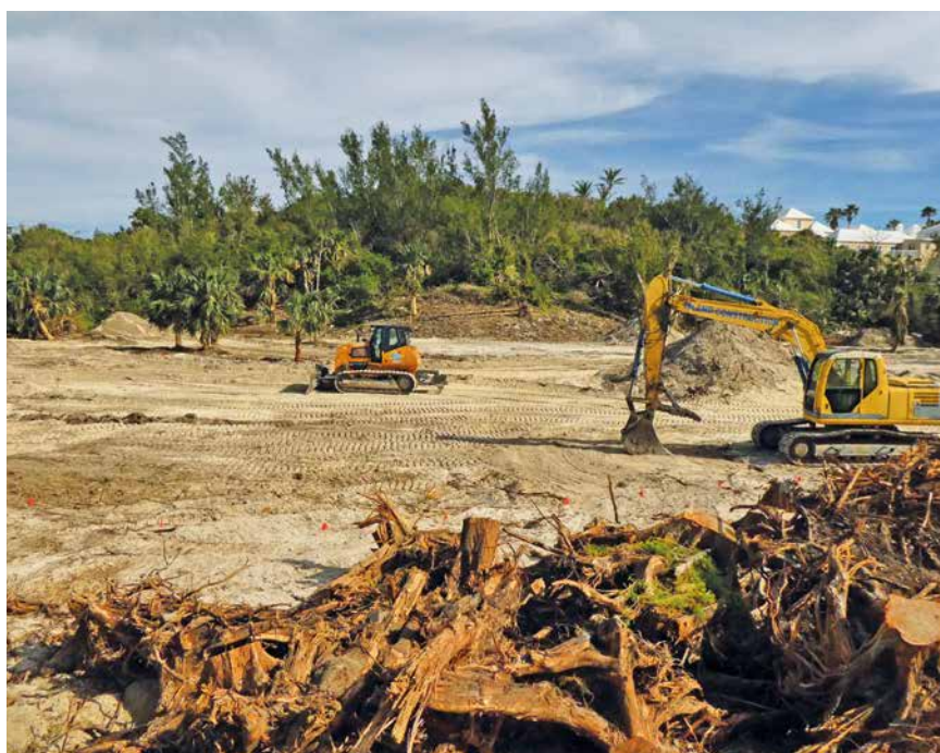
Figure 3a. Site clearing in May 2020 at Eve's Pond, previously filled with sand and colonised by invasive trees.
