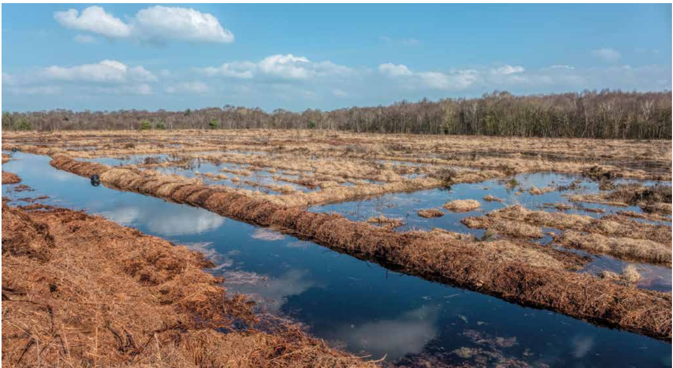
Figure 2. An area of the National Nature Reserve being restored by bunding peat into cells with pipes installed to direct excess water into other areas. The restoration is part of a £5 million EU LIFE-funded Marches Mosses BogLIFE Project. Photo: Stephen Barlow.
