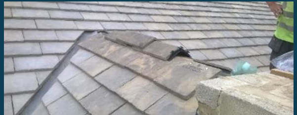
Ridge tiles in situ showing an access gap
