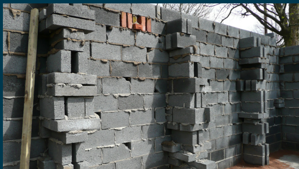
Cavity wall comprising compressed cinder block inner wall with brick outer leaf. Walls deliberately left rough for additional perching/roosting and with deep wall cavities also.
