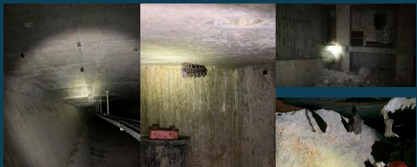
The abutment chambers and connecting tunnels are used by lesser horseshoe bats and other species
