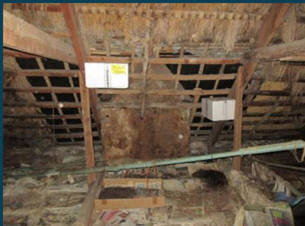
Holne roost: these polystyrene food boxes were placed in the maternity roost. The concentration of droppings shows the boxes are well-used, which makes it easier to clear out any build-up.
