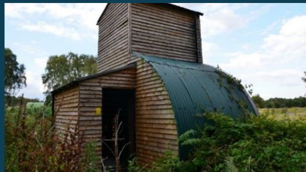
August 2012 – vegetation starting to encroach on bat structure
