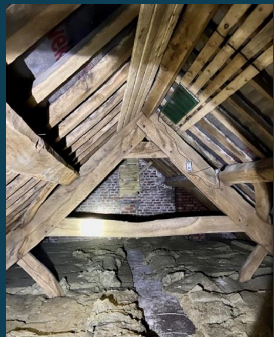
All existing timbers were maintained and droppings retained in the loft space. Interior of roost has additional timber provision and a heating panel (droppings present below this feature).
