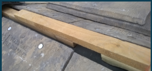
Gaps can be created by using two battens with spaces. In this photo, the ridge roll was omitted (they often contain BRM) and the battens placed directly onto Type 1F 1F bitumen felt. Screws go through the clip/bracket and into the ridge board.
