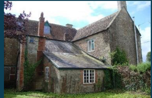
Western view of the farmhouse (mitigation roof void roost on the right of the photo)
