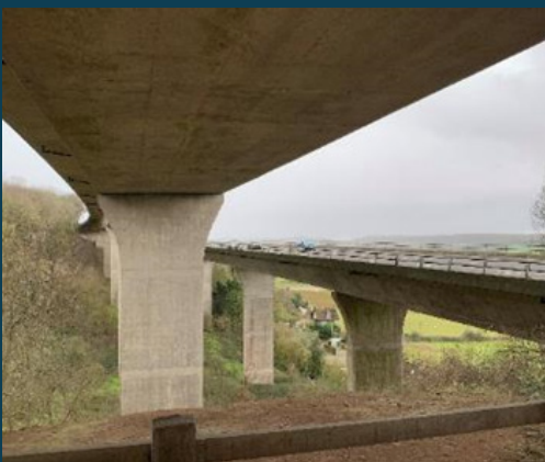
The viaduct has a large void through it and at each end in abutment chambers.
