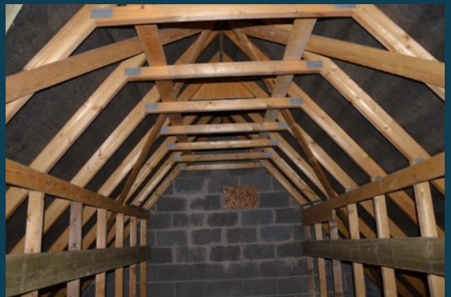
A modified open-plan trussed roof was used with a rough timber ridge board inserted at the apex and an additional false purlin inserted 600 mm above floor level
