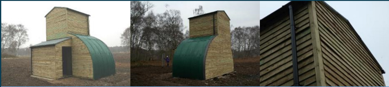
Completed conversion – 2009. Timber wedges (right) were added to create gaps behind the timber cladding
