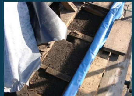
Gutter with lead removed showing droppings
