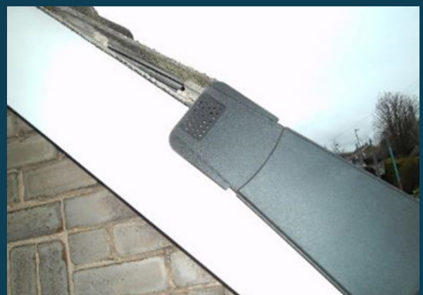
Dry verges are also used along the edges of roofs (again, instead of mortar), shown here without bat adaptations.
