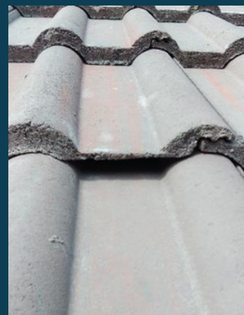
Crevice access created by cutting a notch in the tile to create a gap (20 mm wide and the length of the tile)
