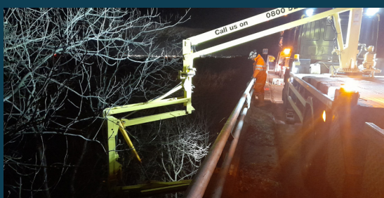
Serious access equipment required
