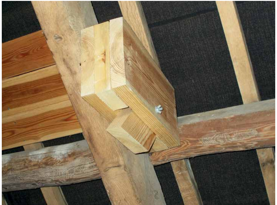
Artificial gappy mortise joint in new loft. Photo credit Andrew Ross.
