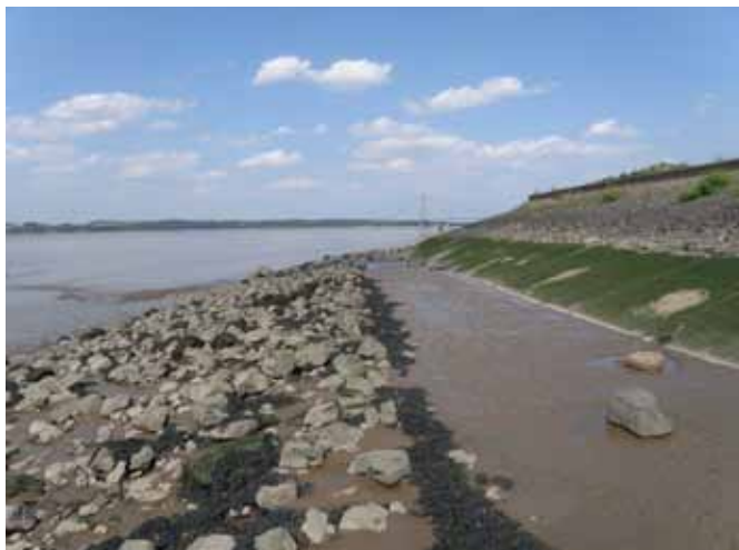
Figure 1. Foreshore at Barton on Humber. In this case, the toe of the sea wall has been extended by about 2 m over several hundreds of metres, reducing the extent of usable inter-tidal and compounding coastal squeeze problems that are illustrated by lowered mudflat heights and exposure of the toe of the wall (thus requiring remedial action).
