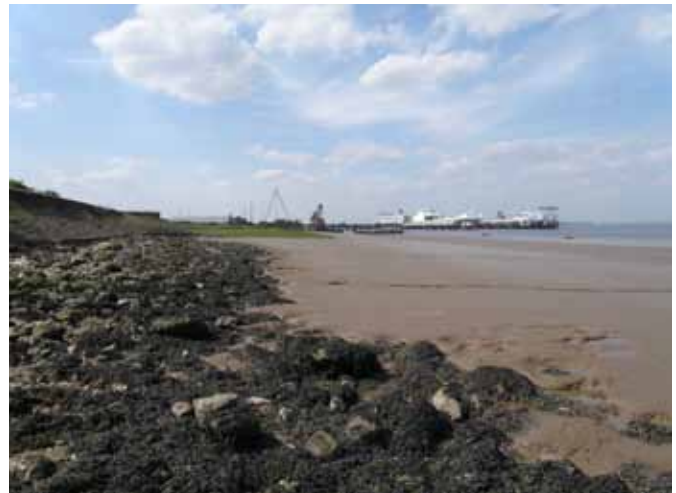
Figure 3. South Killingholme (Humber Estuary) where foreshore lowering is exposing the toes of the sea wall as a consequence of coastal squeeze. Movement of the sea walls into the estuary will exacerbate the problem, leading to further foreshore lowering as well as loss of a footprint within the designated site. Note the extension of the green foreshore where the mudflats about saltmarsh and the wave climate is buffered by energy absorbing saltmarsh. Photo: Roger Morris
