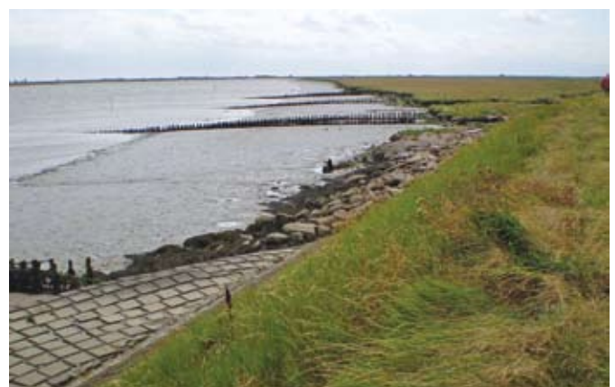
Photograph 4. Armouring at the base of the sea wall at the eastern end of Wallasea Island, Crouch and Roach Estuary, Essex. This illustrates how foreshore recession has led to piecemeal attempts to maintain the integrity of the sea wall.
