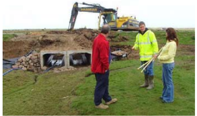
Coastal realignment work in Northumberland undertaken by the Environment Agency can realise conservation benefits
