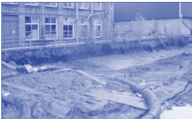
Ferncliffe Road Bund and pumps
