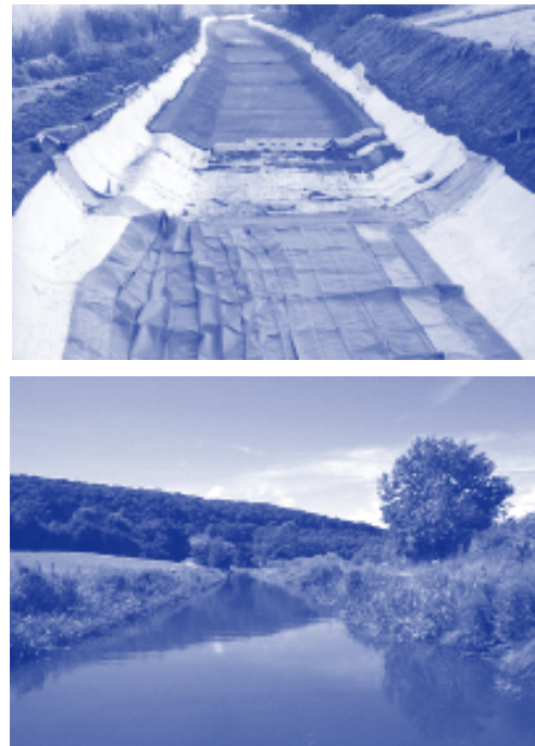
Figure 3: Photographs taken during and 2 years after the construction of the PVC & concrete lining in the Bath Valley.
