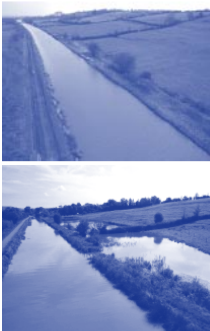
Figure 4: Photographs taken during and 6 months after the construction of the new offside lake & piling works at Sells Green.
